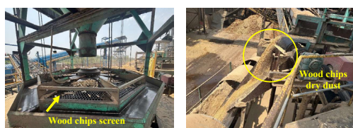
Fig. 2: Wood chip screening and dust recovery for use in boiler
