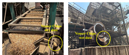
Fig. 1: Veneer chip residue recovery for use in boiler
