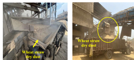
Fig. 3 Wheat straw dust recovery for use in boiler
