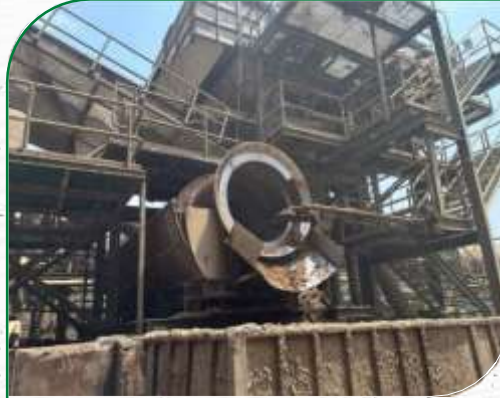
VENEER CHIPS WET DUST DAILY EXTRACTION: 15 TPD
