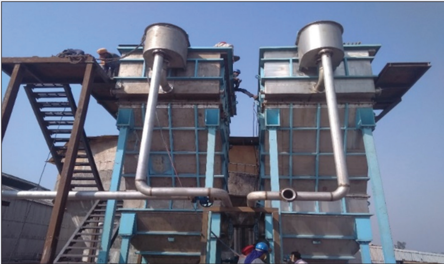
MPS Installed at Kuantam Paper Ltd.
