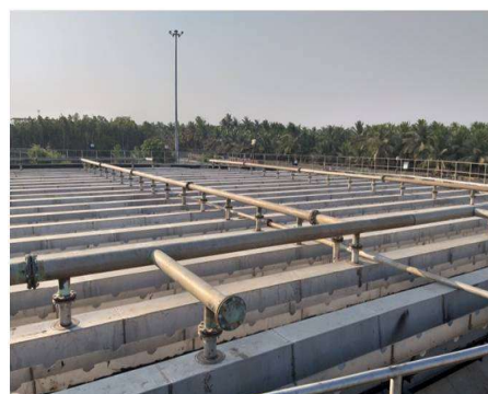
Figure 6 Biogas Collection Pipe line
