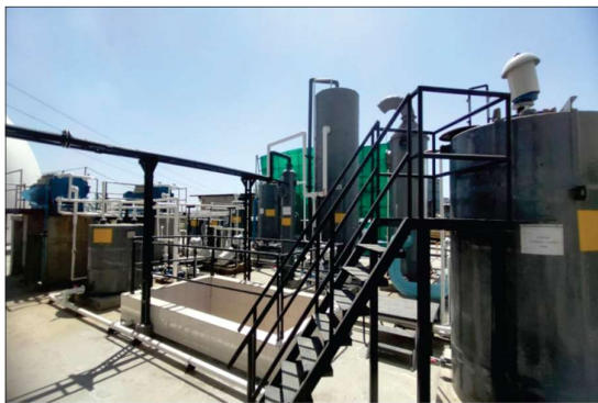
Figure 2: PSA and Scrubber System
