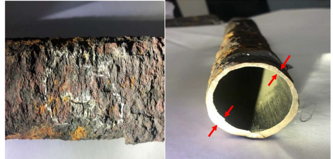
Figure 1 Superheater tube external corrosion and thickness reduction
