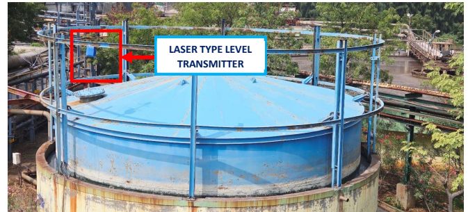
Figure 4: Control system in biogas holder
