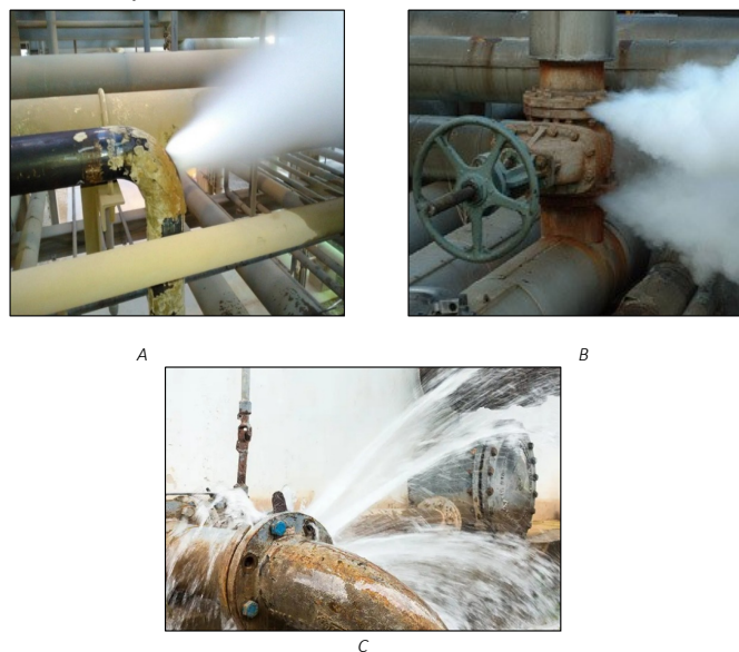
Fig 1. A. Steam Leak from pipeline. B. Steam Leak from Flange of Valve. C. Chemical or water leak from flange of valve.[6]
