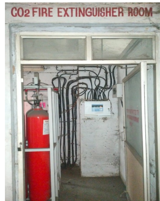
Figure: 17 CO 2 Cylinders Storage Room at TG
