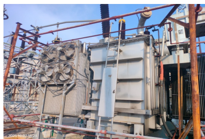
Figure: 1 Transformer with Automatic Water Sprinkling System
