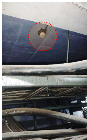
Figure: 9 Smoke Sensor in Cable Alley Room
