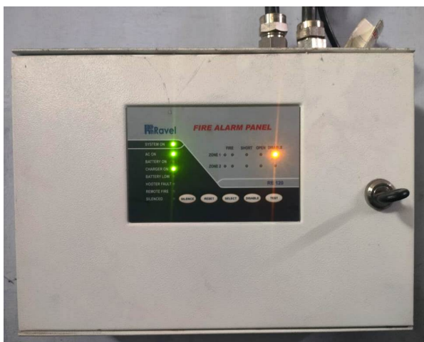
Figure: 12 Fire Alarm Control Panel
