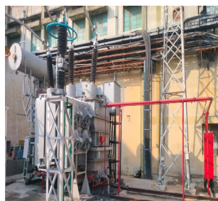
Figure: 4 Transformers with NIFPS
