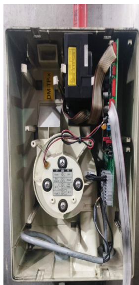
Figure: 20 Components in ASD
