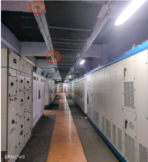
Figure: 6 Low Roof MCC Panel room equipped with APSD
