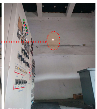
Figure: 11 High Roof MCC with IR Receiver
