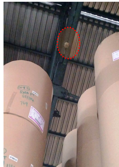
Figure: 21 Smoke Sensor in Reel Storage
