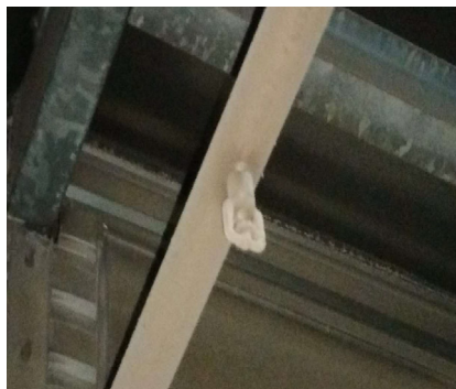
Figure: 15 Water Sprinkler
