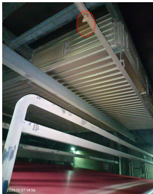
Figure: 13 Water Sprinkler System inside Dryer Hood
