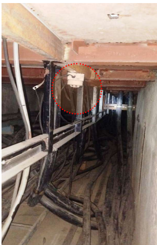
Figure: 8 Smoke Sensors in Cable Trench
