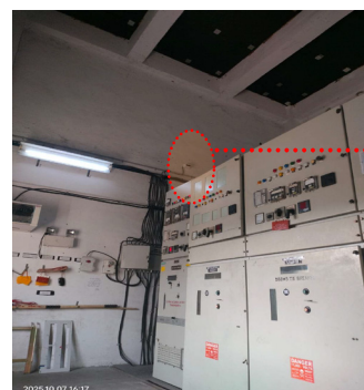
Figure: 10 High Roofs MCC with IR Emitter
