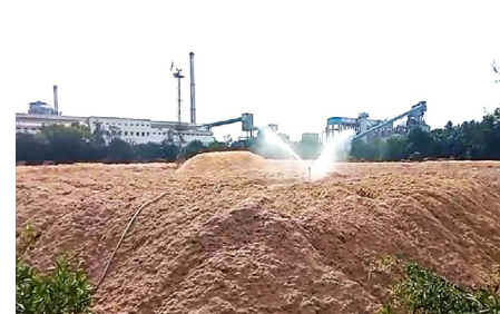
Fig.6 : Sprinkler system -Bagasse yard.
