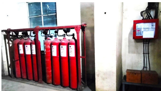
Fig. 4: 16 / 21 MW turbines - CO 2 suppression system.
