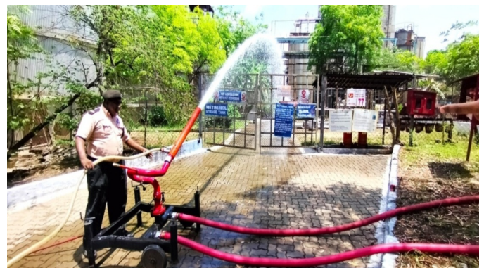
Fig. 10: Methanol Storage Tank – Testing of Water Monitor.
