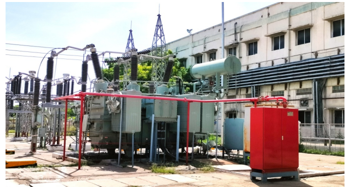
Fig. 5: 11KV Transformer - Nitrogen Injection Fire Prevention system.
