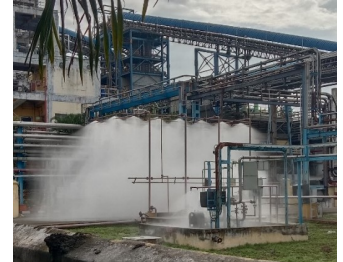
Fig. 16: Methanol tanker unloading sprinkler system
