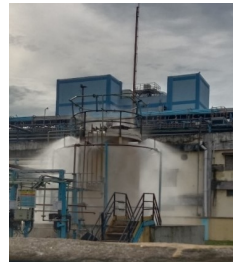
Fig. 15: HSD storage tank sprinkler system
