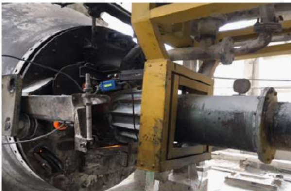
LVHC Gas inlet Pipe line at Lime Kiln for incineration
