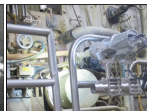
(Fig 3) Jet cut-through Monitoring
