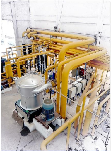
Stock Preparation System
