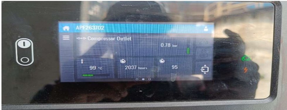
PICTURE OF CONTROLLER UNIT SCREW BLOWERS
