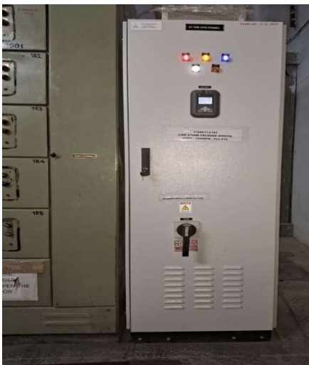
Fig 4 VFD for Limestone crusher
