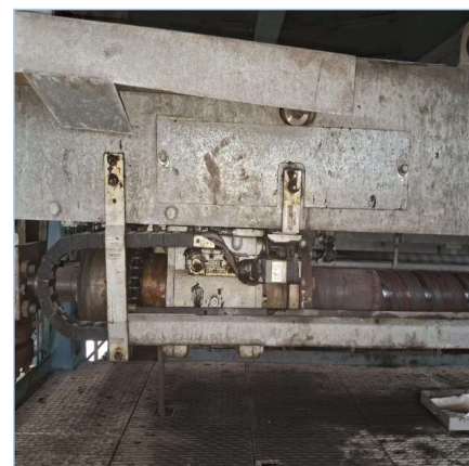
Fig 2. Previous Limit switch in soot blower
