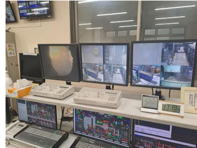
Machine DCS Room
