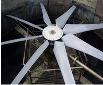
Cooling tower fan with 8 blades
