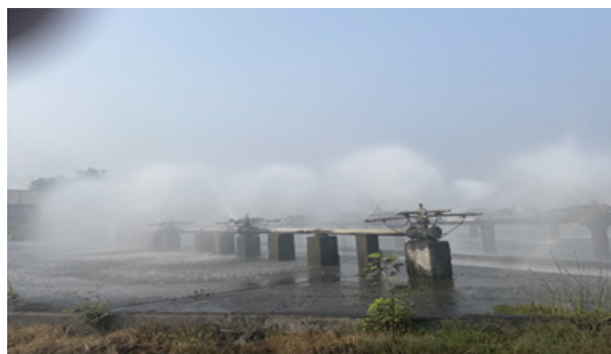
Fig.1 Spray Pond View with water spray from the Nozzles
