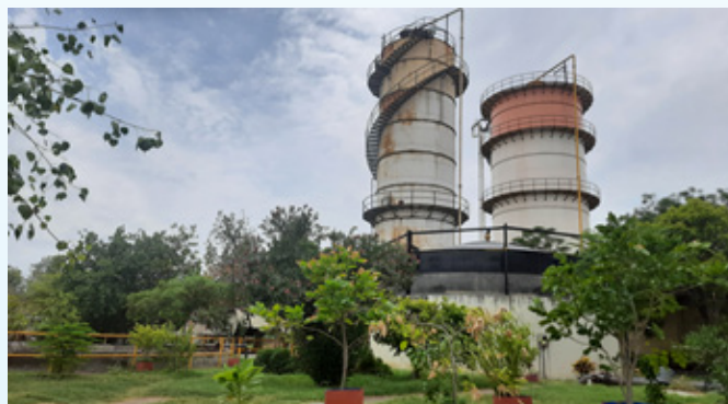
Old and new ULRD Anaerobic reactor
