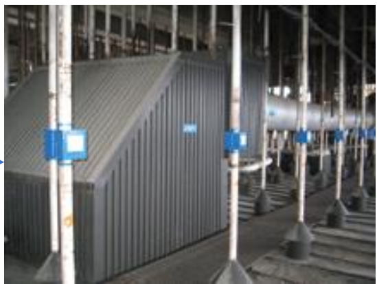
Direct deposit accumulation measurement with Fouling Sensor
