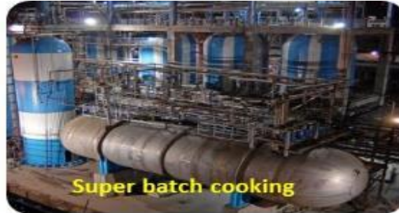
Super Batch Digesters SP. Steam Cons < by 30%
