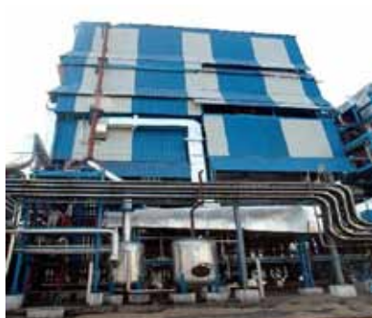
Fig-2A : Coal fired High Pressure Boiler- CPP
