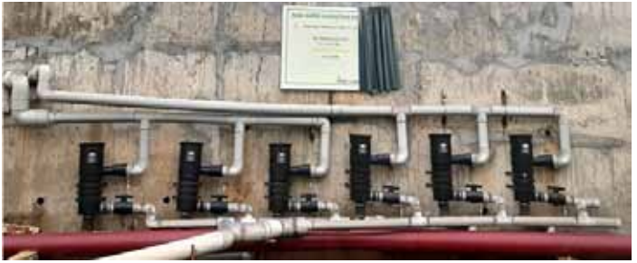
Figure 3: Photograph of the filters of rain water harvesting system
