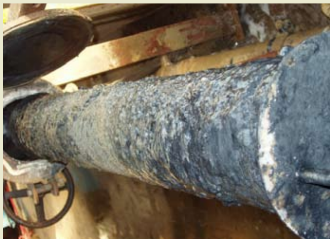
Figure 3. Slime inside shower bar rich of iron sulfide deposit— indication of anaerobic growth
