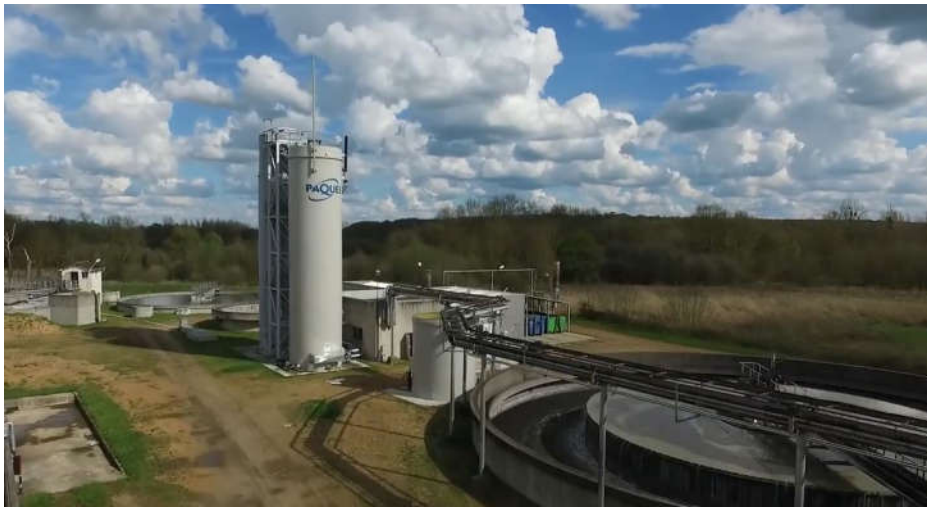
Figure 6. The anaerobic BIOPAQ®ICX reactor at Allard Emballages, France.
