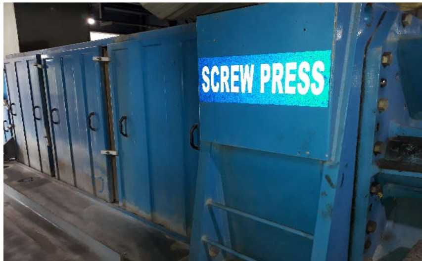
Fig. 6. Photographs of Mechanical de-watering machine (Screw press)
