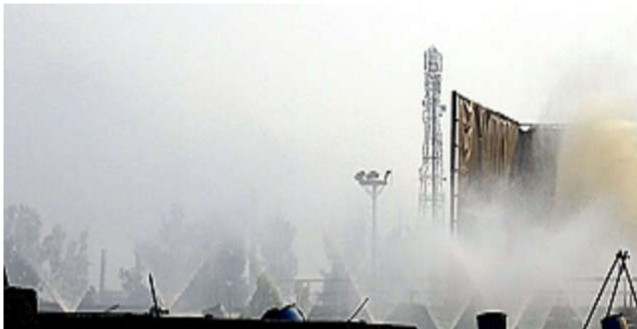
Fig. 10. Mist Aeration System
