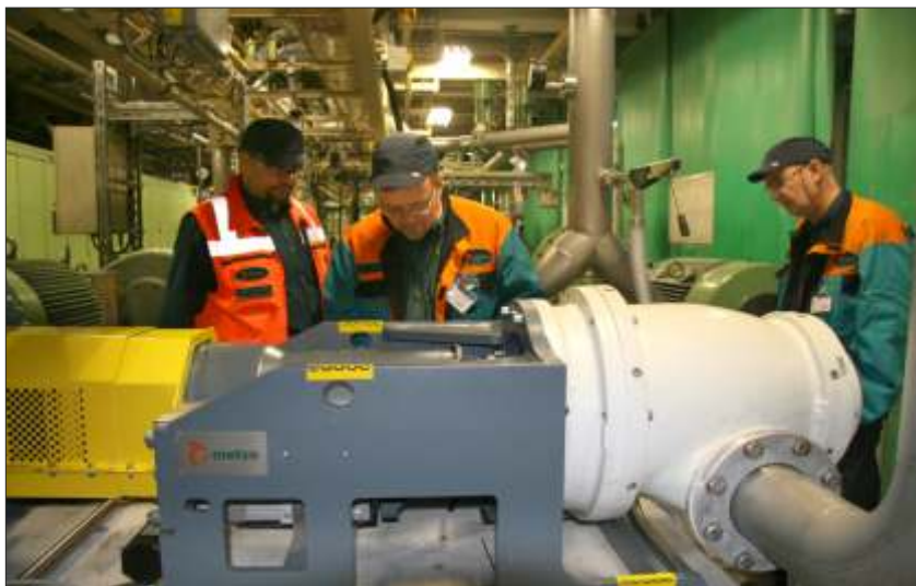
Figure 8. OptiFiner Pro mill installation (Sappi Biberist mill)
