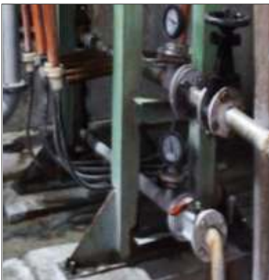
Ecomizer with back flashing
