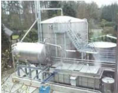
Figure 4: Wastewater tank, DAF and reactor
