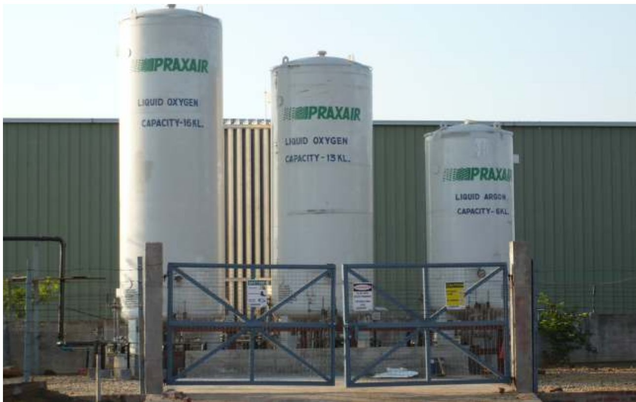
Liquid oxygen storage tanks
