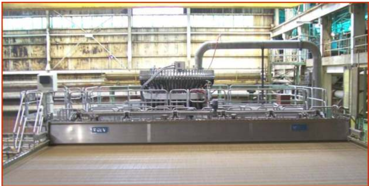
Fig. 3 BTF™ installation on a 9.8m wide linerboard machine
